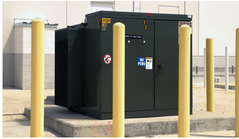
Transformer outside a data center
